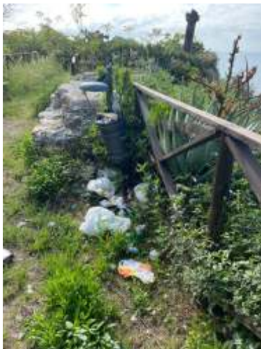
State of decay
